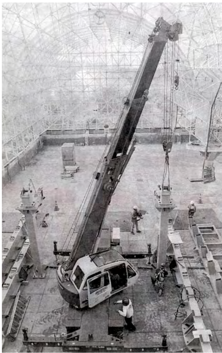
A crane from Parsons Steel Erectors moves a support beam into place inside Biosphere 2. Big equipment had to squeeze into the glass structure.
